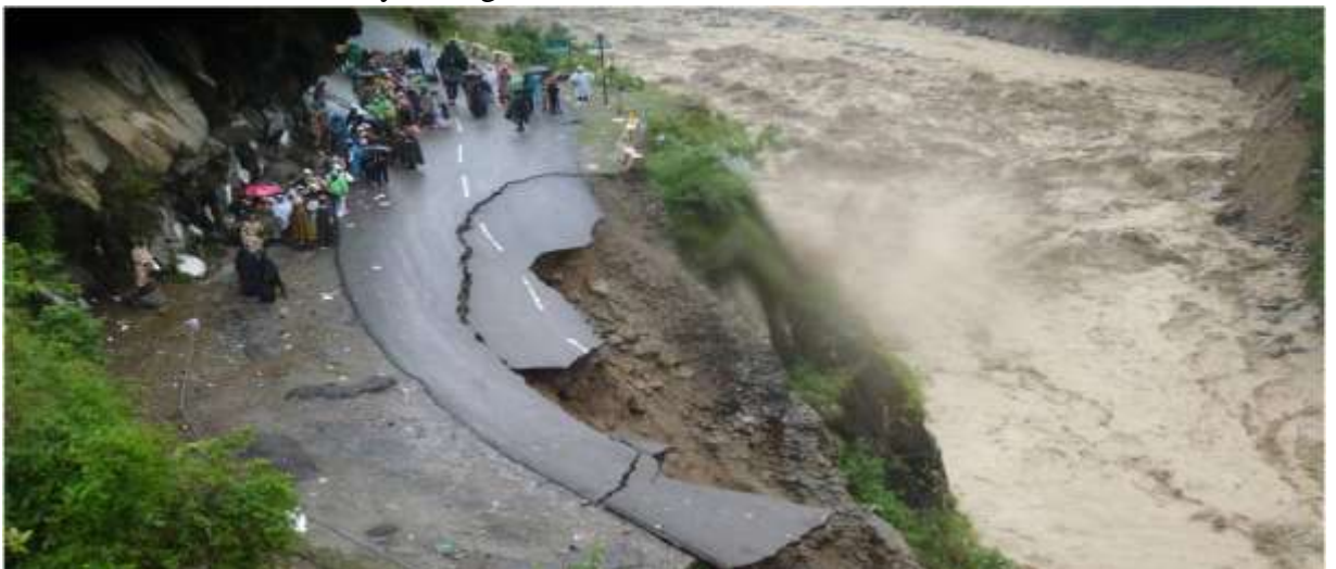
Figure 5: Damages in Chamoli District
